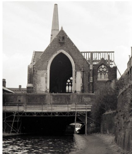
The Church of the Messiah, Broad St., Birmingham being demolished in 1978. Looking towards Gas Street Basin.
